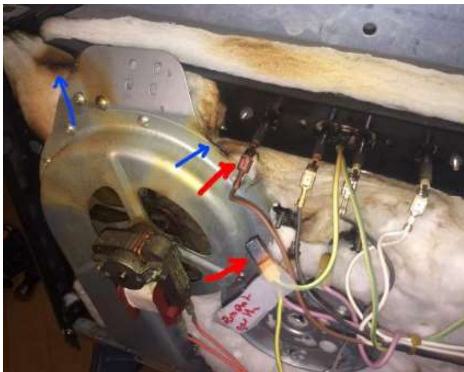
Figure 14: Faulty risks in electric
