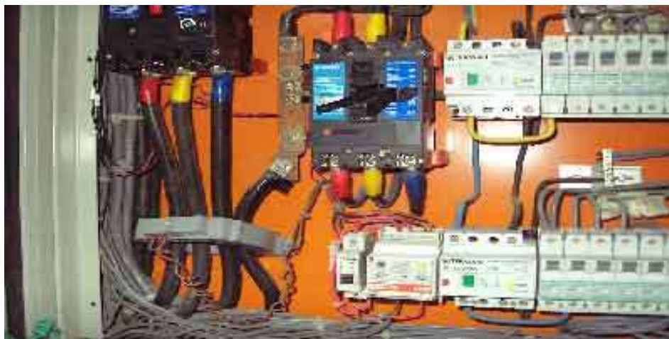
Figure 9: industrial main switch
