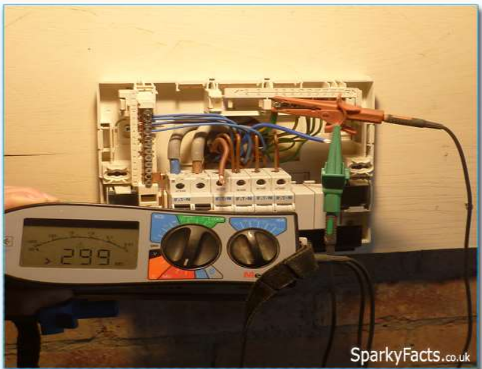
Figure 323 Insulation Resistance test sequence
