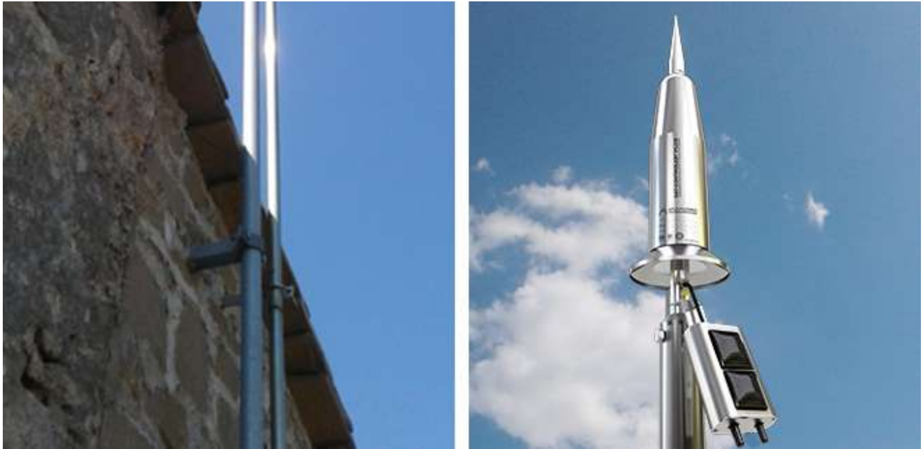
Figure 53: Lightning rod image
