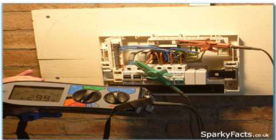
Figure 322 Insulation Resistance test sequence
